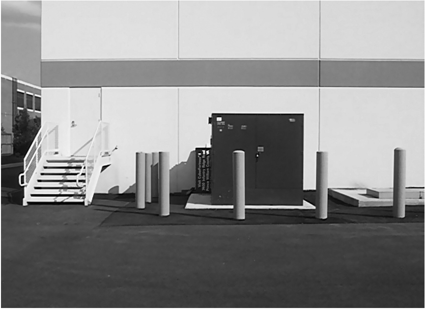
Figure 9.19 Illustration of a Transformer Located Outside a Facility and Protected by Bollards.
