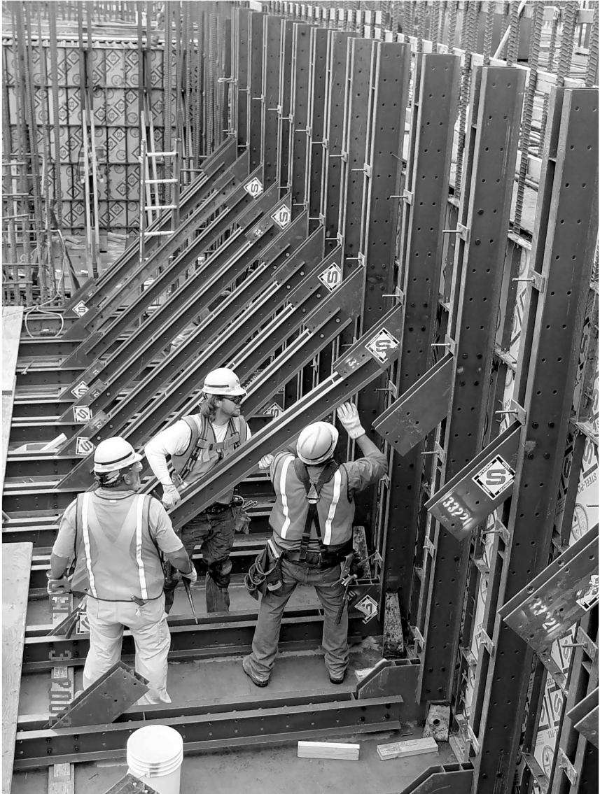
Figure 6.9 Photo of Carpenters Setting Concrete Formwork for the High Level Waste Facility Pit Walls. Source: Bechtel Corporation.
