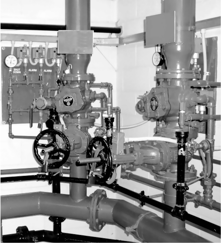
Figure 9.25 Photo of a Fire Sprinkler Control Valve Assembly Installation. Source: Wikipedia.
