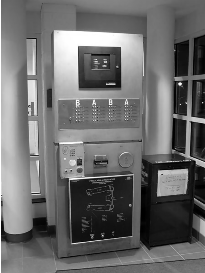
Figure 9.33 A Siemens MXL Fire Alarm Control Panel (top) and Graphic Annunciator (bottom) for Potomac Hall, at James Madison University. Source: Wikipedia, Photograph by Ben Schumin.
