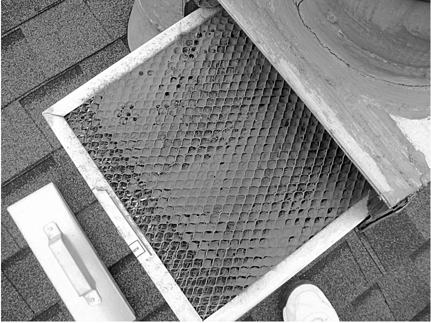
Figure 9.15 A Photograph Showing a Clogged Filter that has been Removed From an AC Unit. It is critically important to change filters periodically to minimize pollution and improve indoor air quality.
