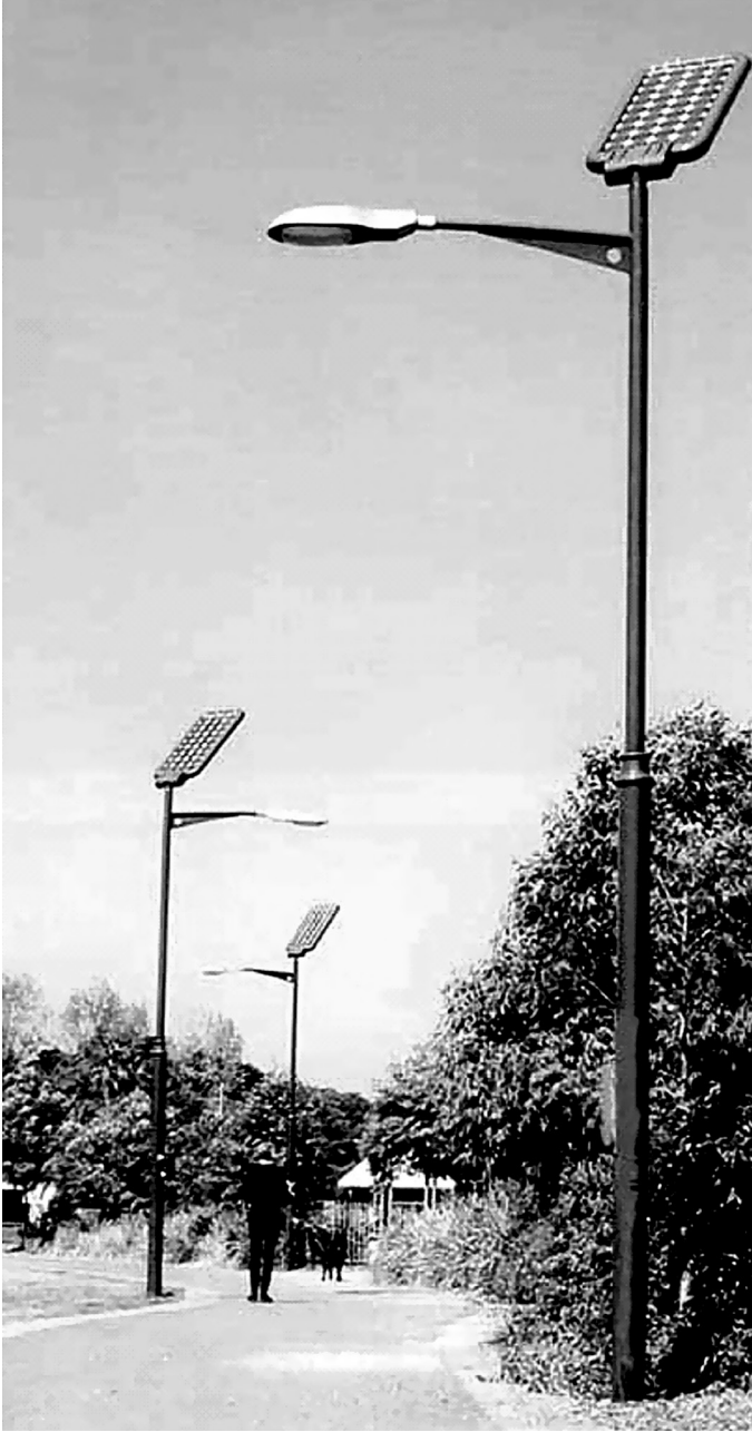
Figure 9.21 Example of Solar Power LED Street Lighting With Automatic On-Off, Lasts for 4–5 Nights After Fully Charged. Source: Hankey Asia Ltd.
