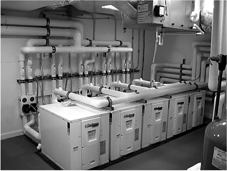
Figure 9.6 A Residential Geothermal Heat Pump System. Source: Climate Heating and Cooling, Inc.
